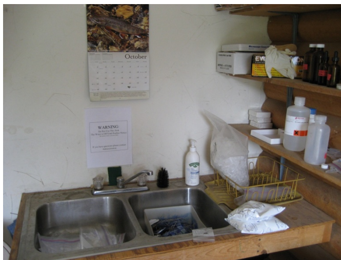
Photo 1-5 Non-functional sink used for storage in Murray Building
