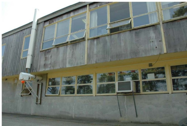
Photo 1-1 View of the exterior of the main laboratory building at existing Bigelow Laboratory campus
