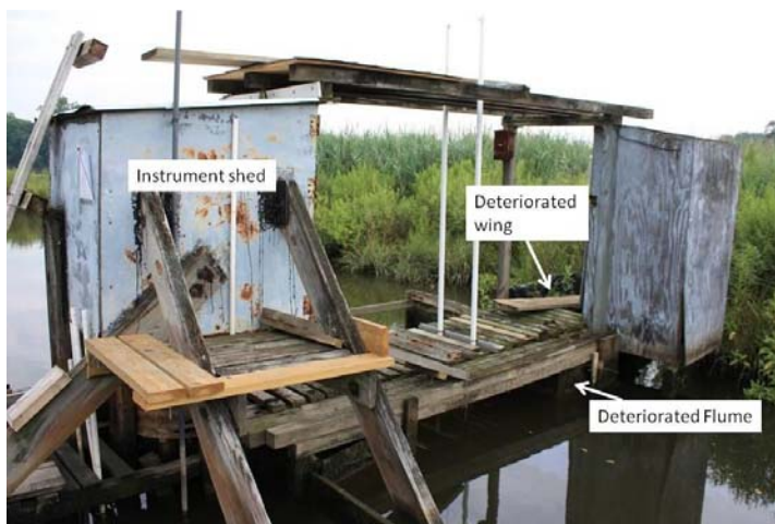
Photo 1-3 Existing, deteriorated flux station
