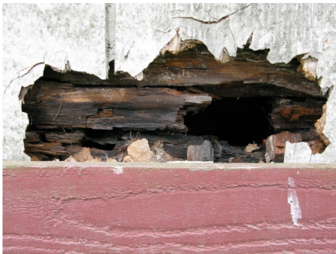
Photo 1-7 Rotting wall in existing NWIC laboratory building
