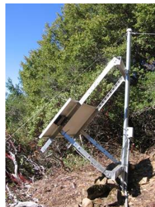
Photo 2-4 Ground-mounted solar panels on six-foot pole
