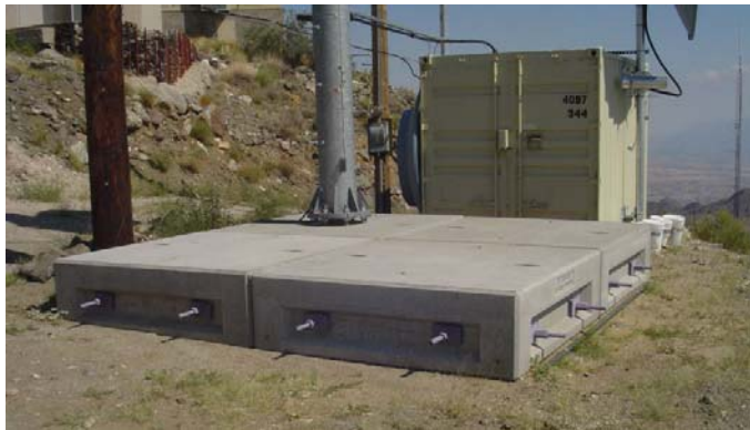
Photo 2-11 Example of above-ground cell block foundation, similar to what is proposed at Anderson Mesa
